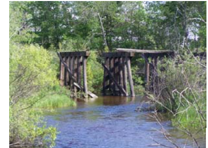
Greater Thompsonville Area - Remnants of the old Pere Marquette railroad bridge over the Betsie River still stand today.
